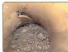
Broken Pipe With Soil Infiltration
