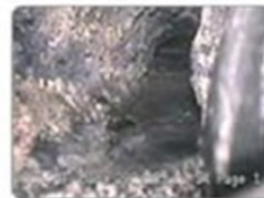
Grease Coated Pipe With Restricted Flow
