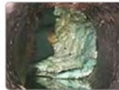
Grease Covered Root Mass
